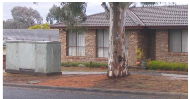
This main electricity box is very dangerous and will affect the occupants' health. Placing a Ba Gua mirror above or on the front door will relieve some tension in the relationship but will not protect from all the EMF (electro magnetic field radiation) affecting health.
